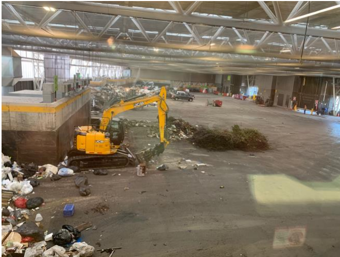
Figure 2 - At the Wallingford-Fremont transfer station, this image is of the dumping floor.
